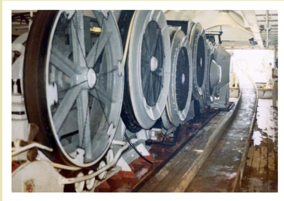
C S Alert 'V' Sheave Cable Engine with Repeater By-pass Trough, 1966
